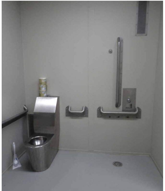
Accessible cell shower and toilet
