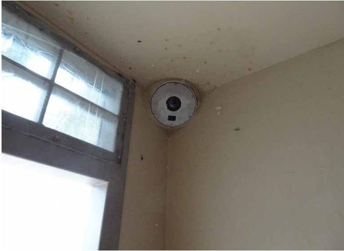
CCTV camera inside cell
