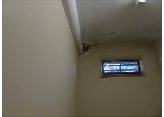
7 wing assessment cell ceiling mould
