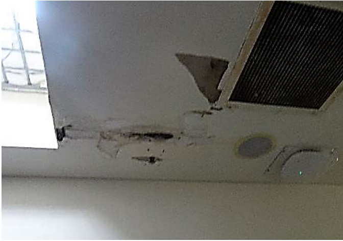
Peeling paint in Sector 3 accommodation
