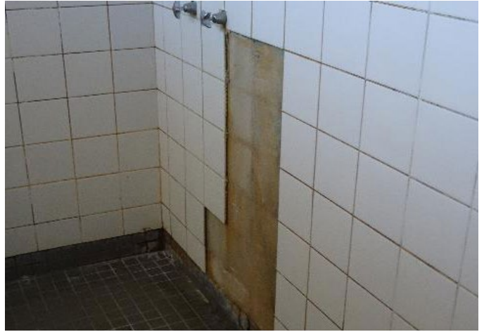
Shower in an accommodation unit
