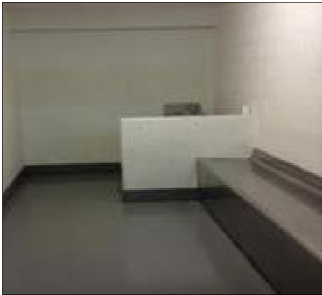
A toilet privacy barrier
