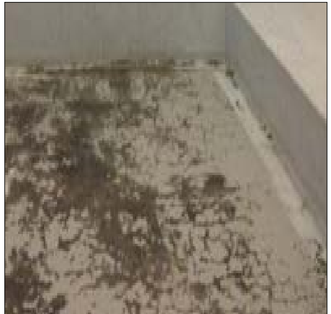
Cell floor requiring repainting
