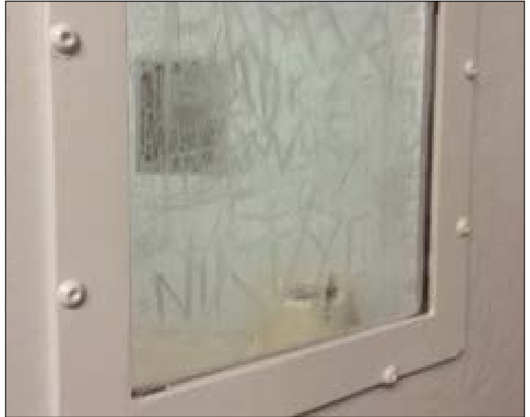
Example of damage on cell door window
